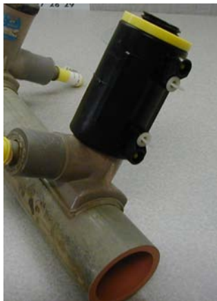
A COMPLETED ELECTROFUSION OF ALDYLA TAP TEE USING KEROTEST REPAIR KIT P/N 72770515
