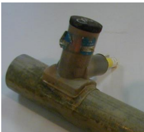
Aldyl-A Tapping Tee with a leaking cap
